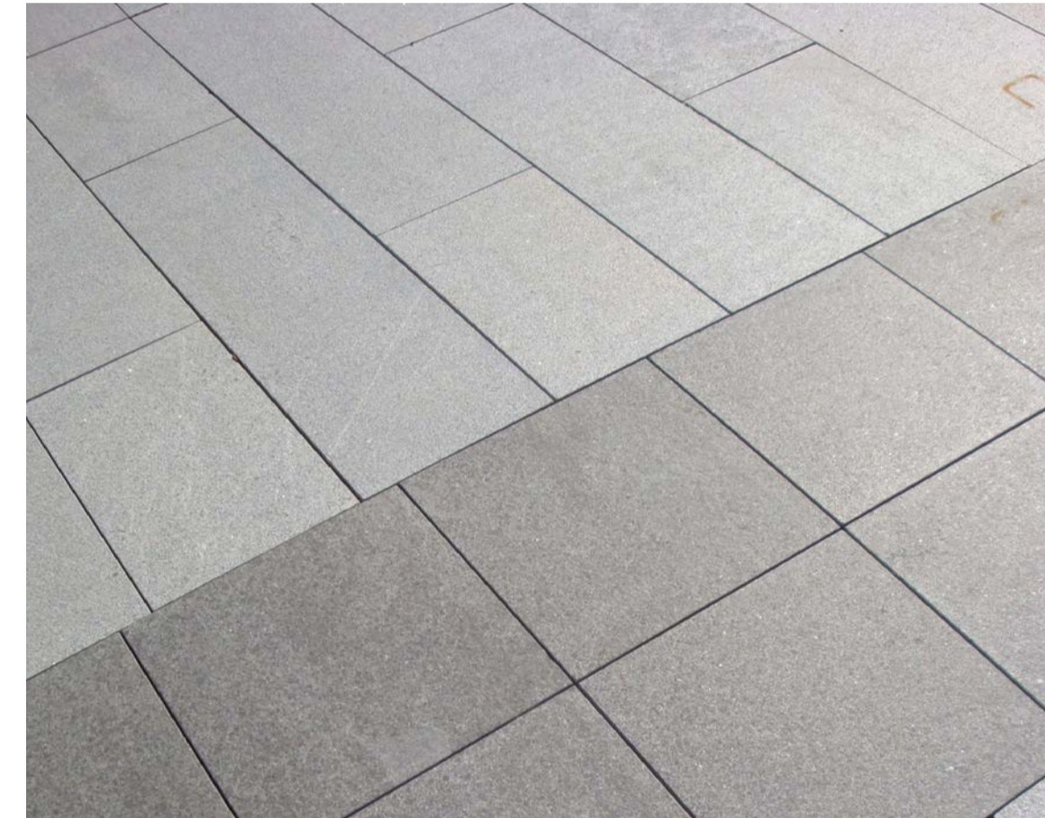
Granite paving, varying stone colours*
